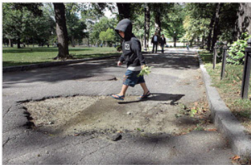
The Boston Common is no stranger to wear and tear. Traces of the disrepair -- missing bricks, uneven pavement, and cracked concrete -- are scattered throughout the grounds.
